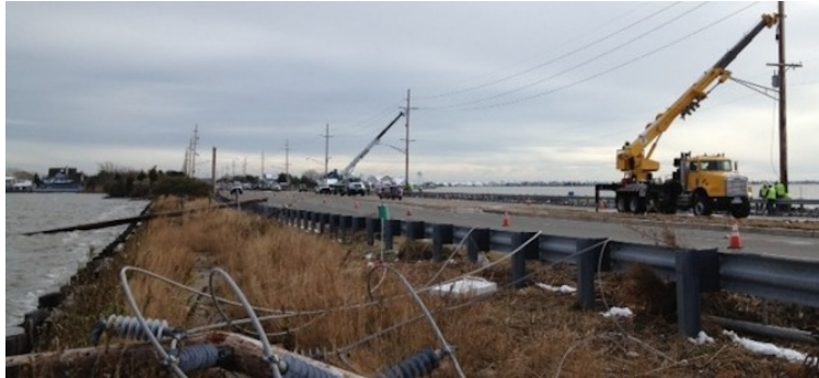
Utility crews at work in Seaside Heights, N.J., after Superstorm Sandy. Photo credit: Western Area Power Admin via Flickr
