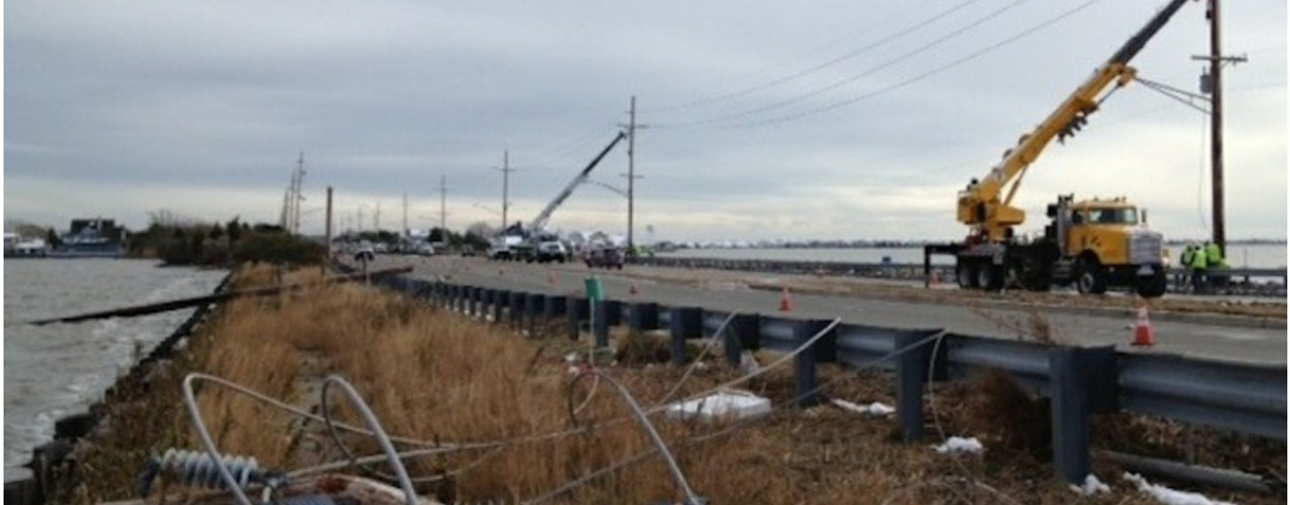
Utility crews at work in Seaside Heights, N.J., after Superstorm Sandy. Photo credit: Western Area Power Admin via Flickr
